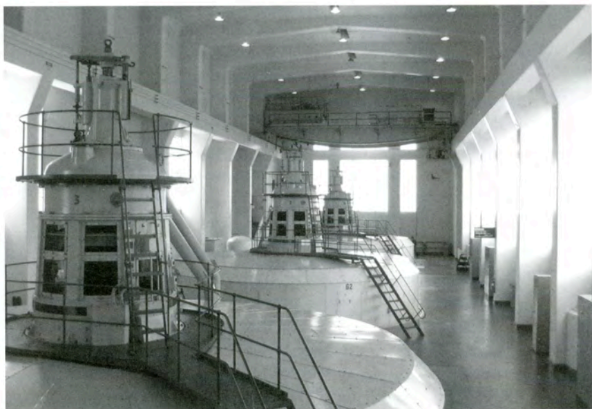
Arapuni Power Station, New Zealand Brian Rice
